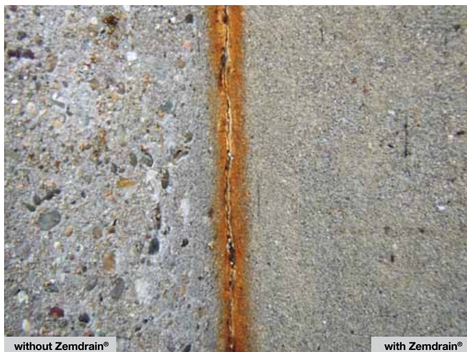
Picture 3: Concrete surfaces: Right side: External wall, surface was cast using Zemdrain® Left side: Spillway wall, surface was cast without using Zemdrain®
