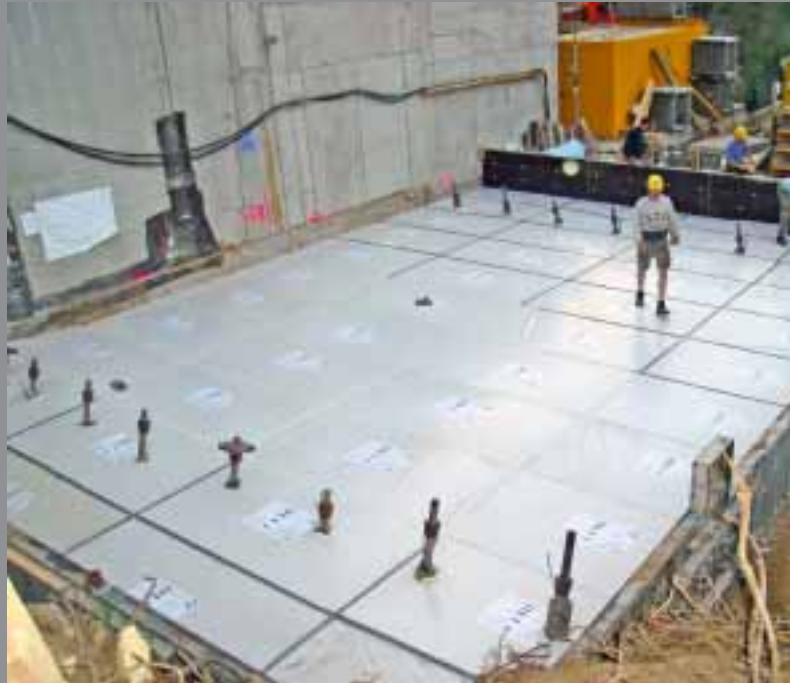
Void formers on existing tunnel floor Void forming layer for the new floor slab to be constructed on
